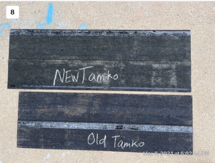
The build of the shingles are not the same.
