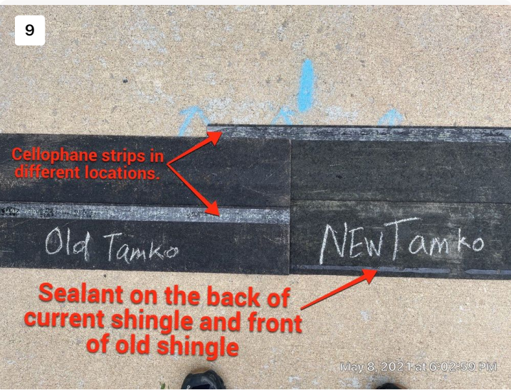
The cellophane on the discontinued shingle is placed differently compared to the current shingle.
